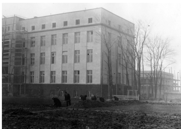
Figure 7. The building of the scientific laboratories of the Radium Institute – finishing works (from the collections of the National Digital Archives)
