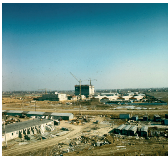
Figure 29. The construction of the new seat of the Institute of Oncology in Ursynów, the late 1970s (from the collections of the editing office of the MSCNRIO)
